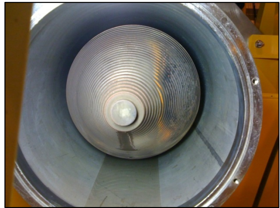
Figure 5: Klystron collector showing traces of overheating (2010).
